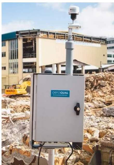
Figure 5.1: Dust Control Monitoring Equipment (Illustrative Only)
